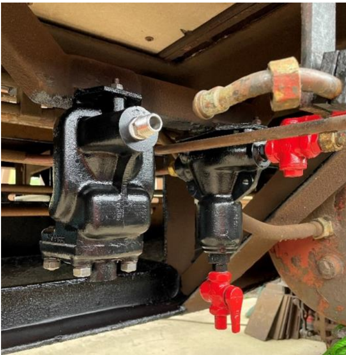
Overhauled air filter/strainer
